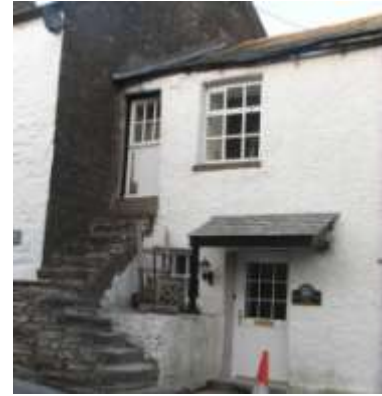
No fascia board or roof overhang Guttering fixed directly to wall by hangers and brackets
